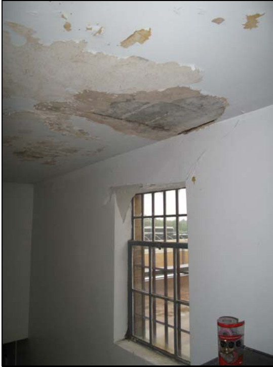
Old water damage on the 4 th floor ceiling.
